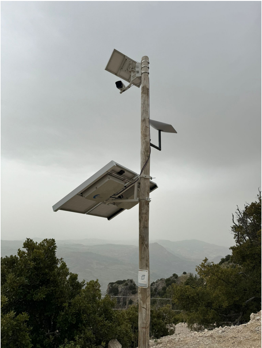
Fig 4-5 One of the five stations of the videosurveillance system
