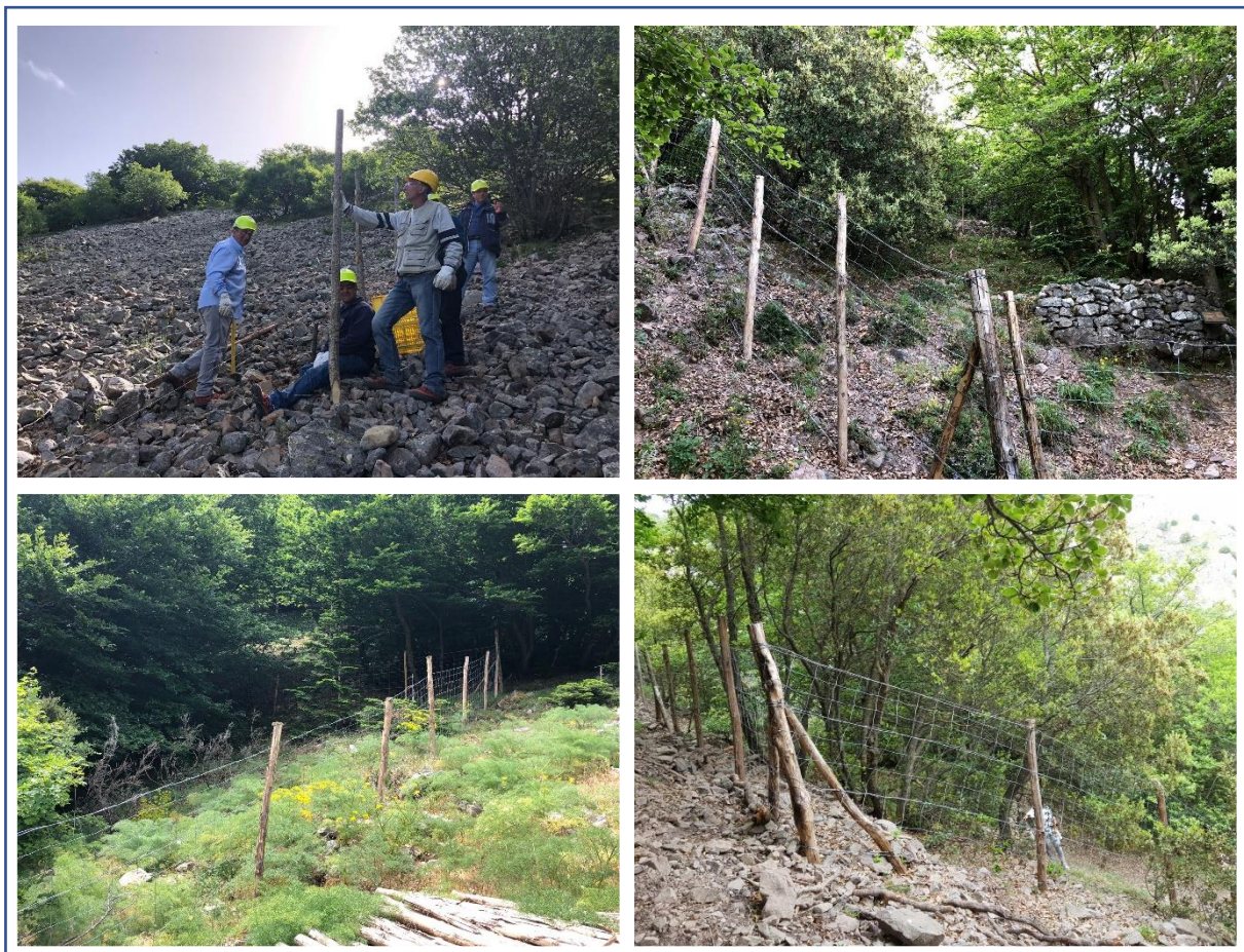
Fig.6. Insertion of poles to the ground (above and left) and fences installed on different kind of terrains.
